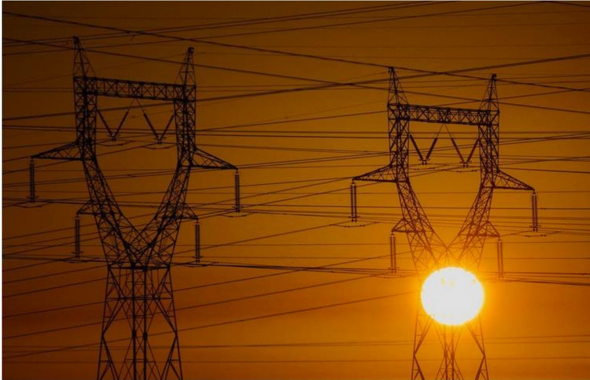
Electrical power pylons of high-tension electricity lines are seen at sunset in Saint-Folquin, near Gravelines, France, November 29,
